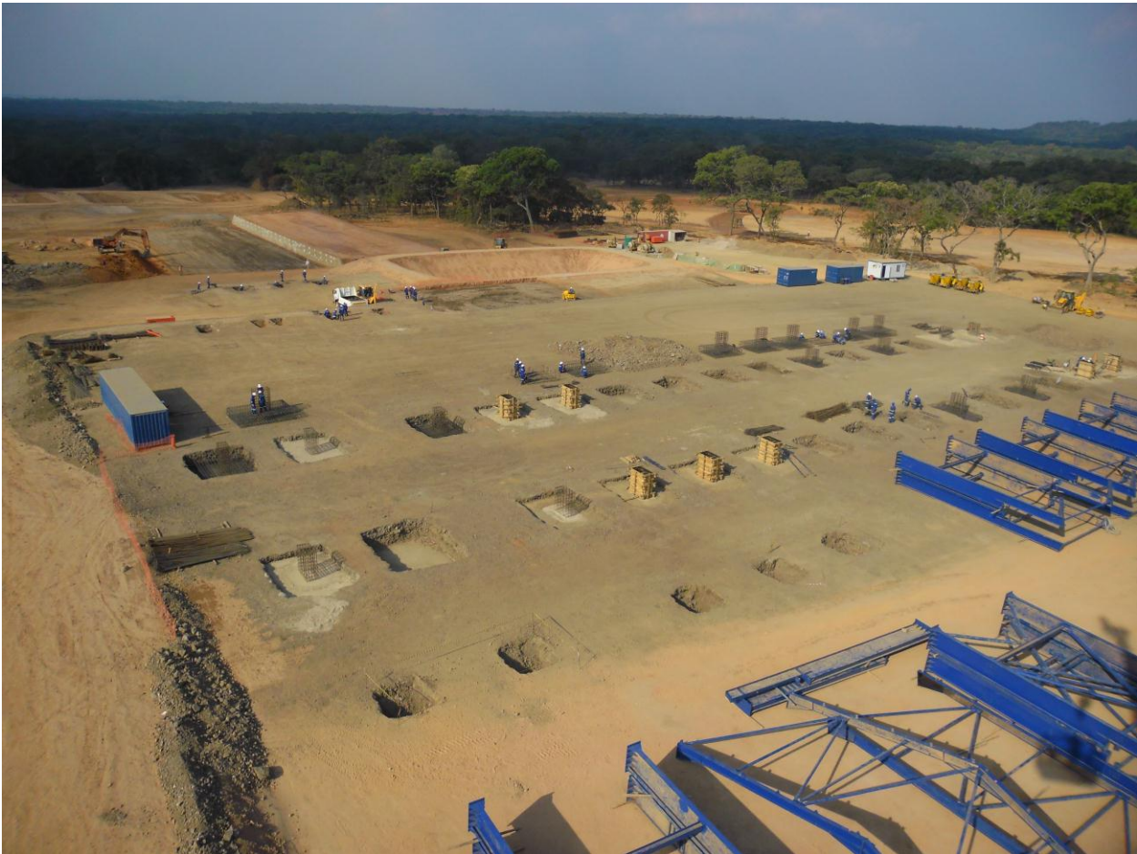
Major steel on site in preparation for erection of the electro-winning facility
